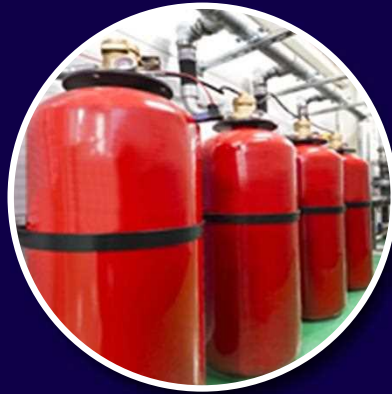
GAS SUPPRESSION SYSTEM
