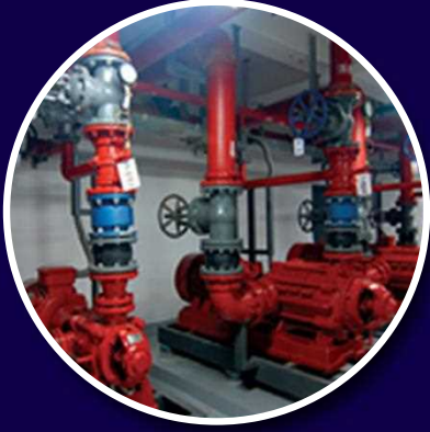
FIRE PROTECTION SYSTEM
